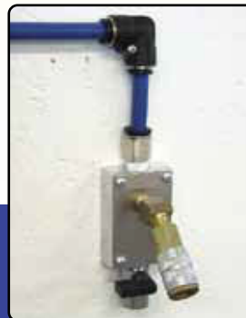
Surface Mount Air line is mounted to wall
